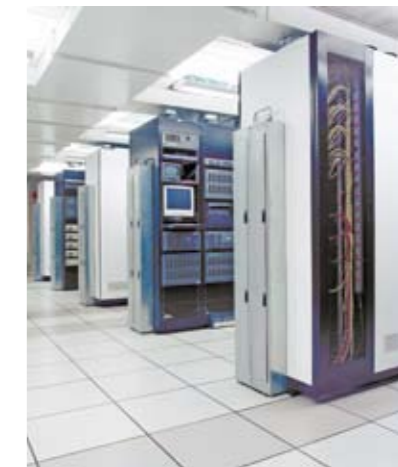
Data Centre – Back-up Power
